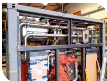
Exhaust after treatment and Heat Recovery during workshop build on a LEAP CHP
