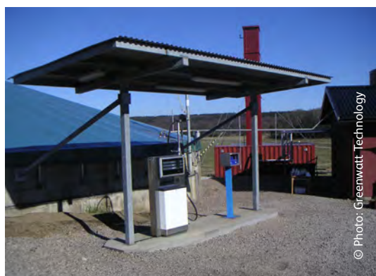
Figure 40: Small-scale biomethane on-farm refuelling station, Sweden
