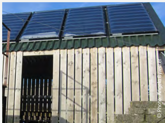
Figure 30: Solar thermal on anaerobic digester building.
