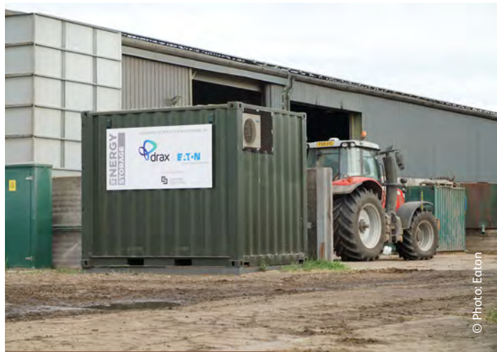
Figure 35: On-farm battery storage
