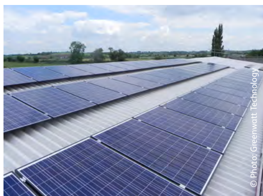
Figure 32: Roof-mounted solar on an agricultural building
